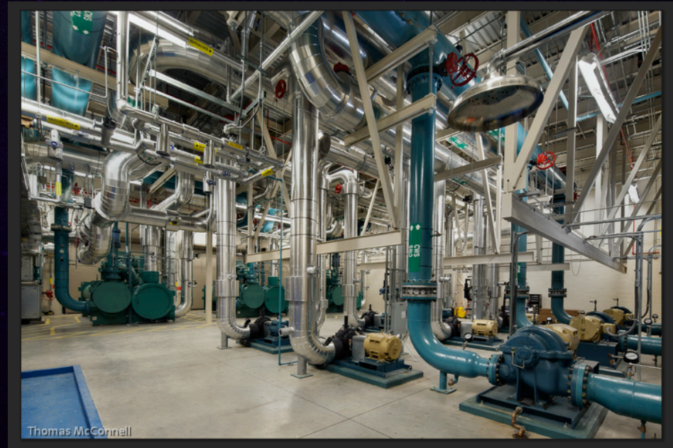
TACC Machine Room Chilled Water Plant
